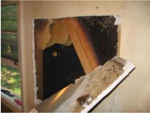
Drywall had to be removed to access the honey bee colony in this wall.
