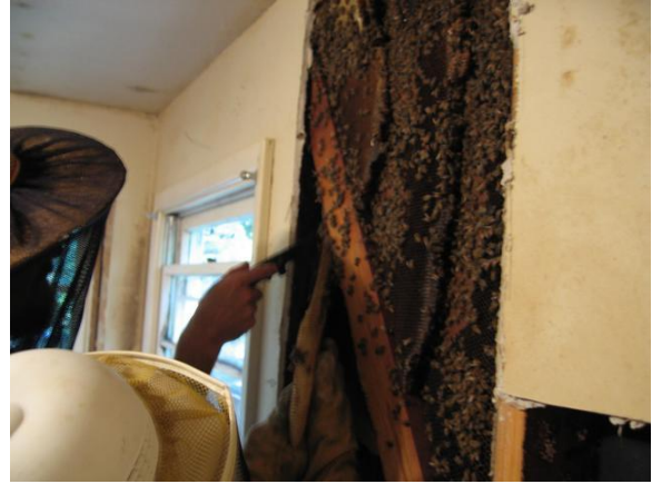
A nice-sized colony in the wall of a house.
